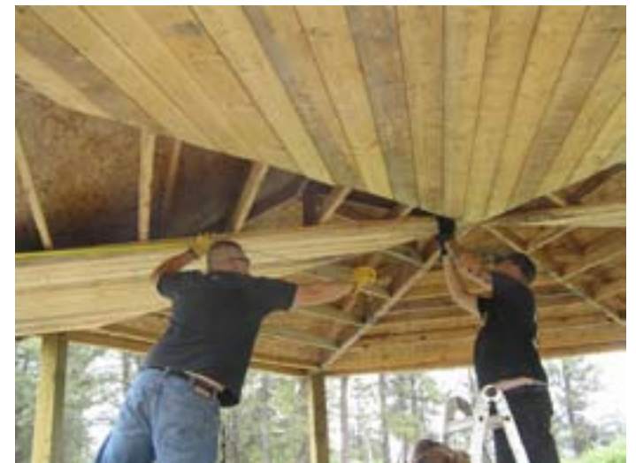
The Veterans Corps and students from SCC constructed the bulk of our last EE shelter (SR)
